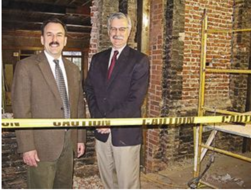
Sales and marketing director Tom O'Gorman, left, and general manager Tom Petot show off some of the reconstruction work at the landmark Exeter Inn that will transform the old restaurant and bar into a two-level, state-of-the-art facility. Diana Paquet photo
